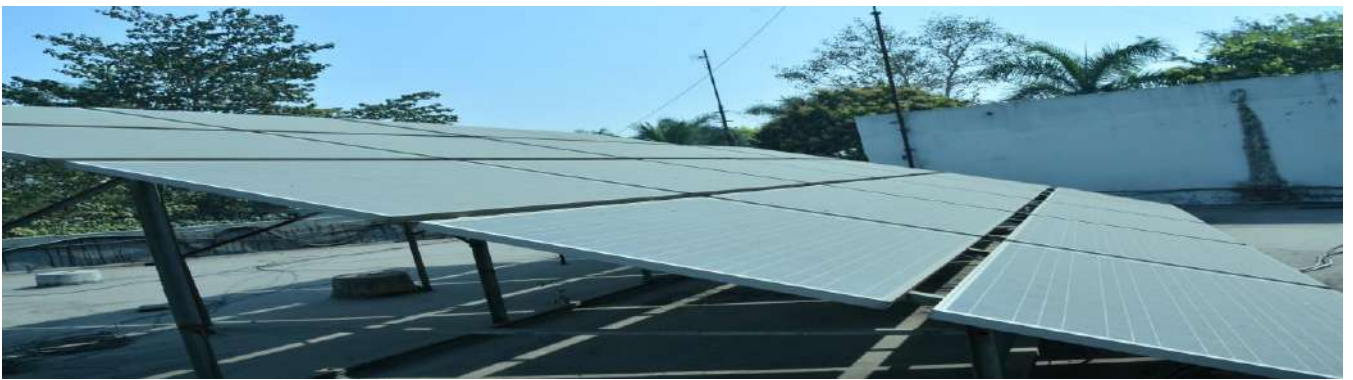
SOLAR PANEL AT SODEPUR AREA VOACTIONAL TRAINING CENTER
