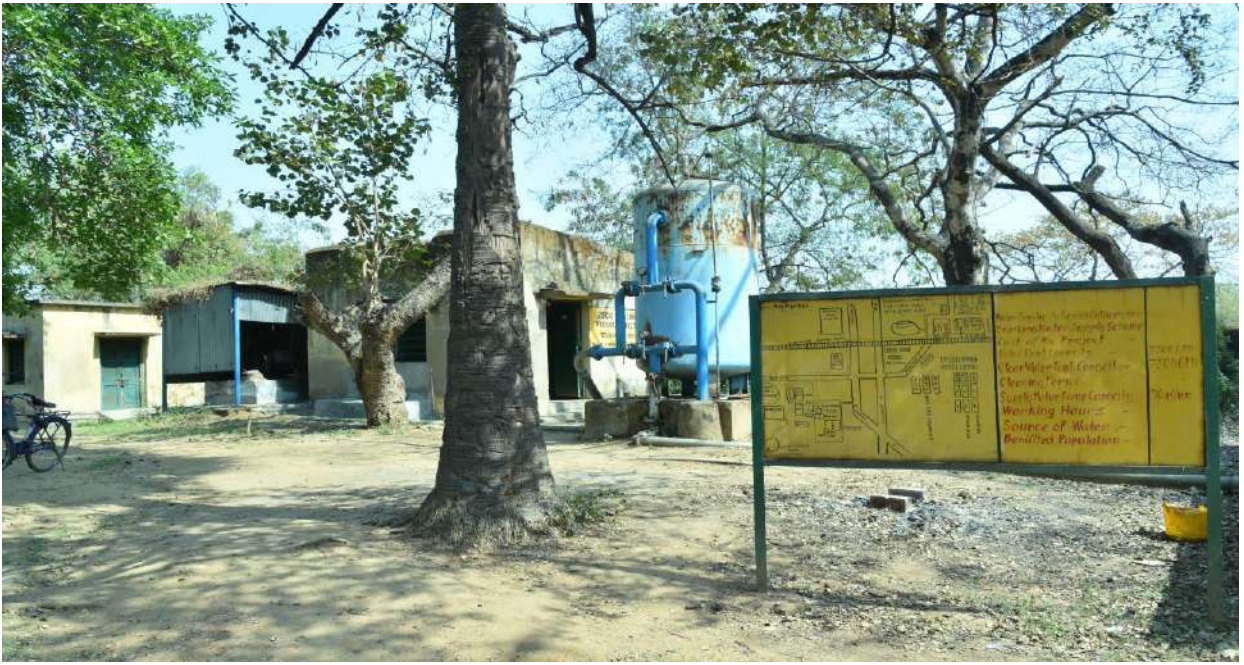
PRESSURE FILTER AT BEJDIH COLLIERY
