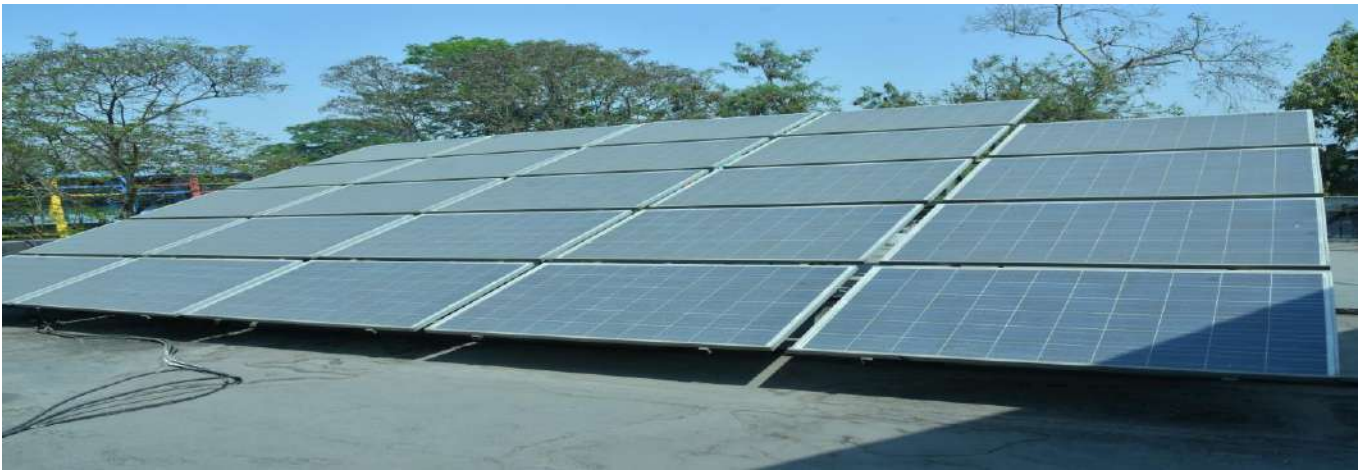
SOLAR PANEL AT SODEPUR ARE OFFICE
