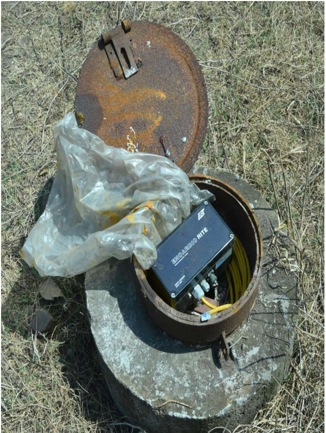
PIEZOMETRIC BOREWELL ALONG WITH AUTOMATI WELL RECORDER AT BHAMARIA IN PARBELIA
