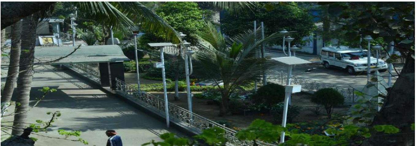
SOLAR LIGHTS AT SODEPUR AREA OFFICE
