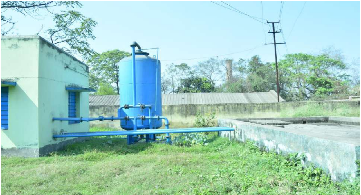
PRESSURE FILTER AT MITHANI COLLIERY
